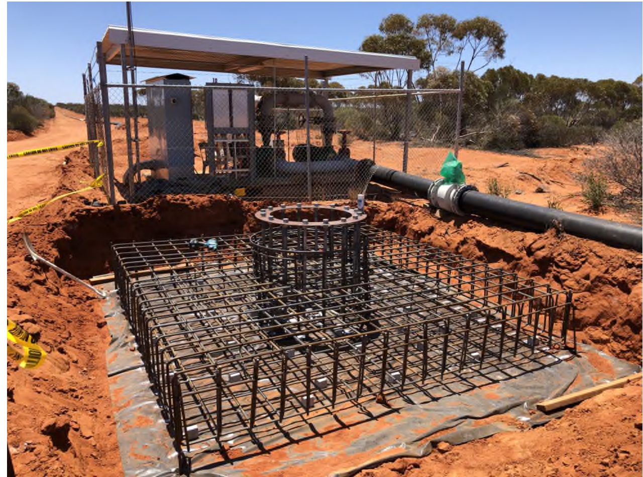
Davyhurst Process Water Supply Footing for Process Water Telemetry Monitoring System Being Installed at Transfer Station
