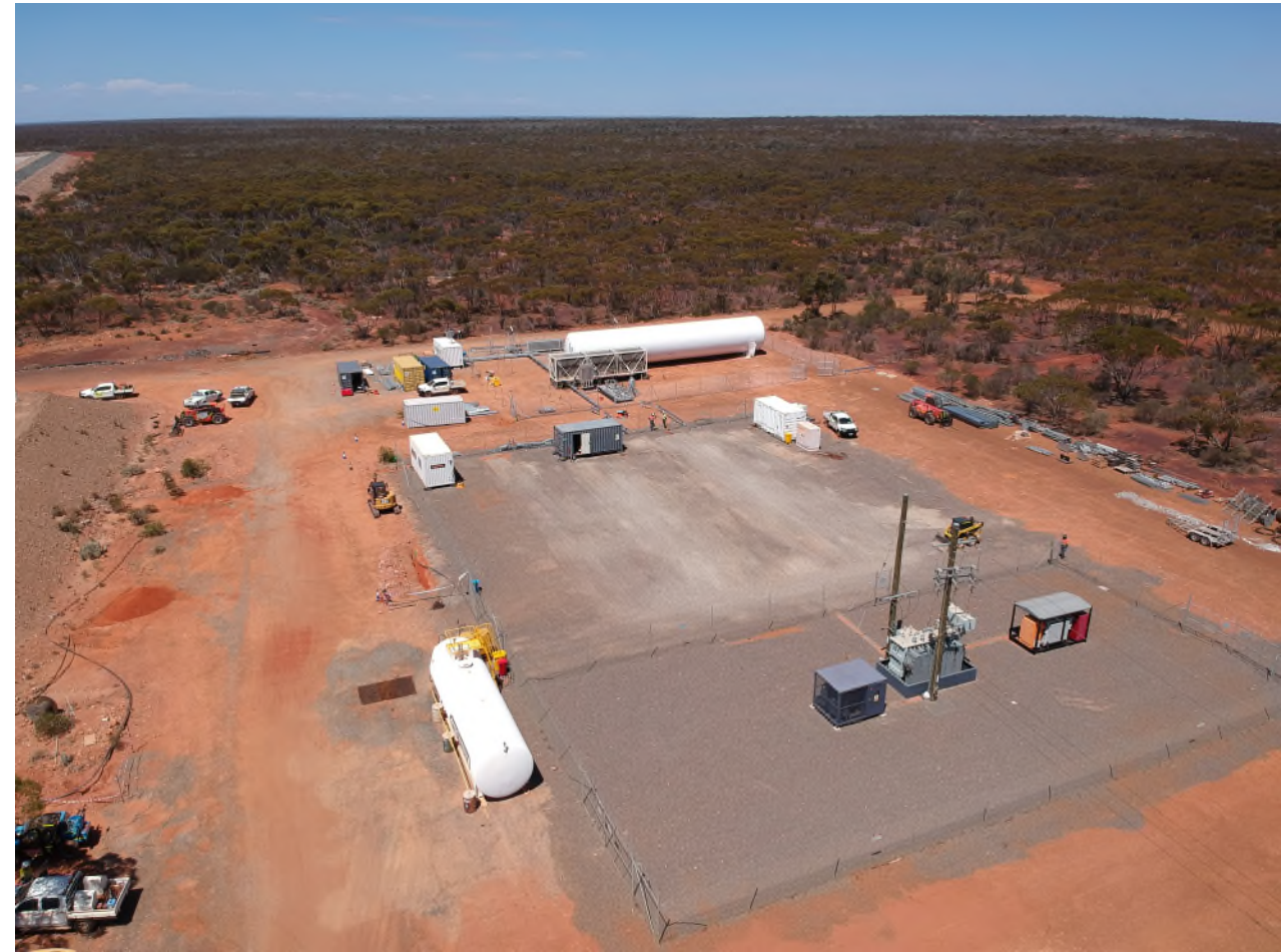
Davyhurst Power Station Preparation for Installation of LNG & Diesel Engines in Progress
