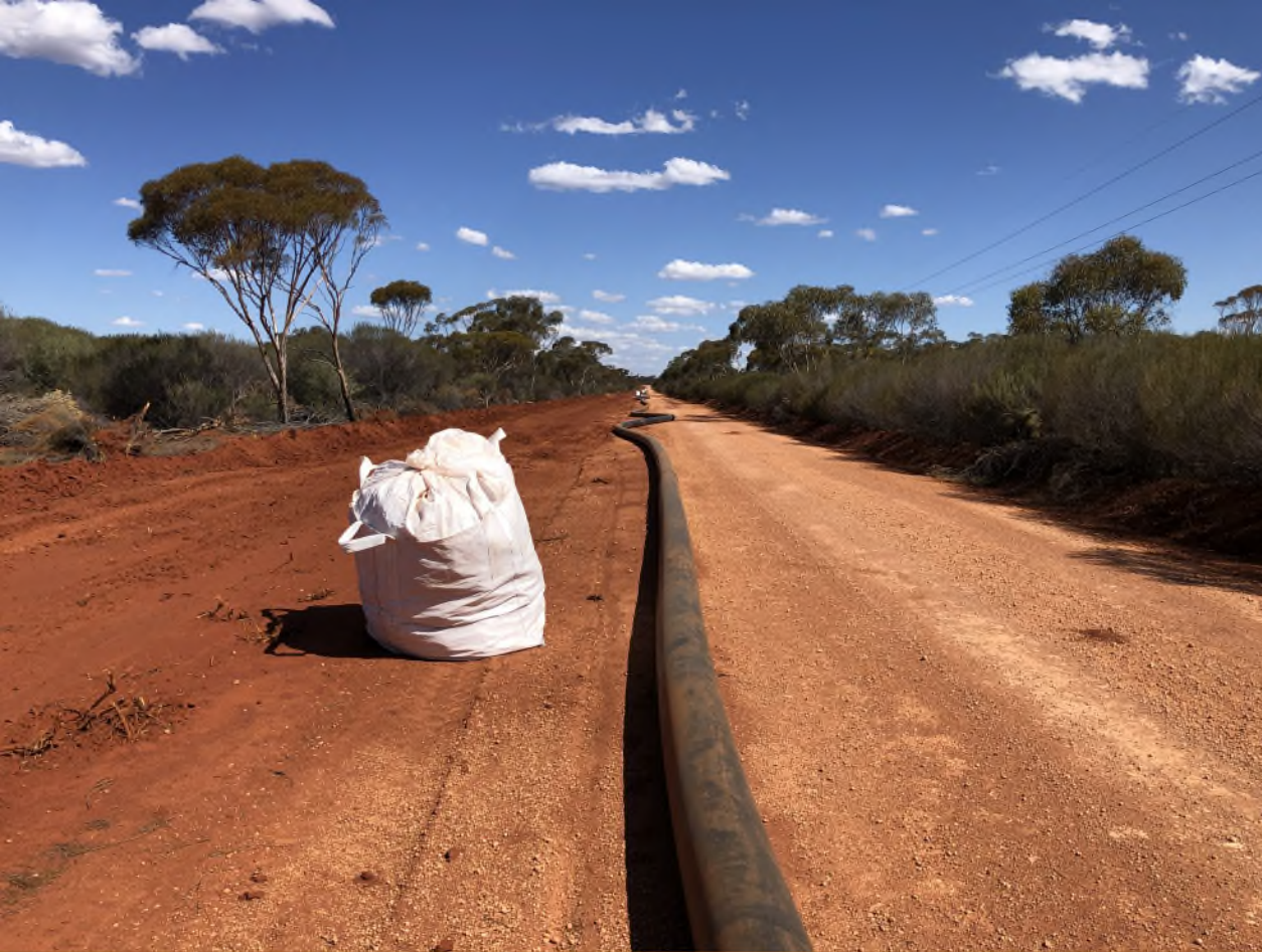
Davyhurst Process Water Supply Process Water Pipeline Firebreaks Re-established and Area Cleaned Up
