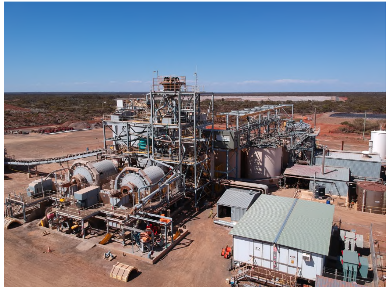
Davyhurst Process Plant Grinding, Gravity & Leach Circuit
