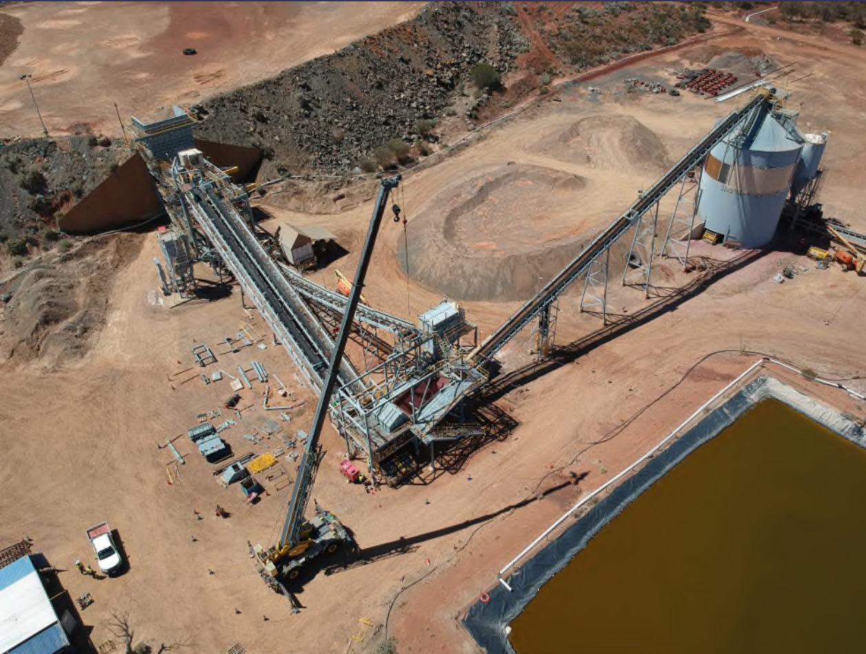
Davyhurst Process Plant Installing Structural Steel at Product Screen Station & Carrying Out Structural Repairs to Fine Ore Bin
